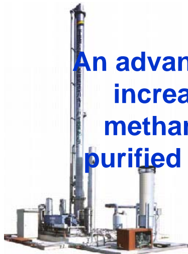
Purification of methane gas
